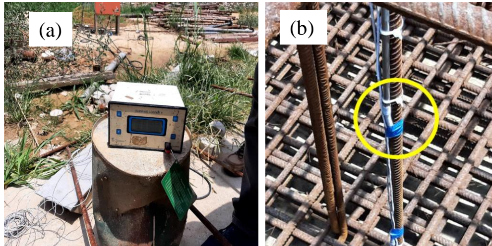
Fig - 4: (a.) Sensor Data Logger used at site (b.) Temperature Sensor embedded in raft reinforcement at core location (L1)
