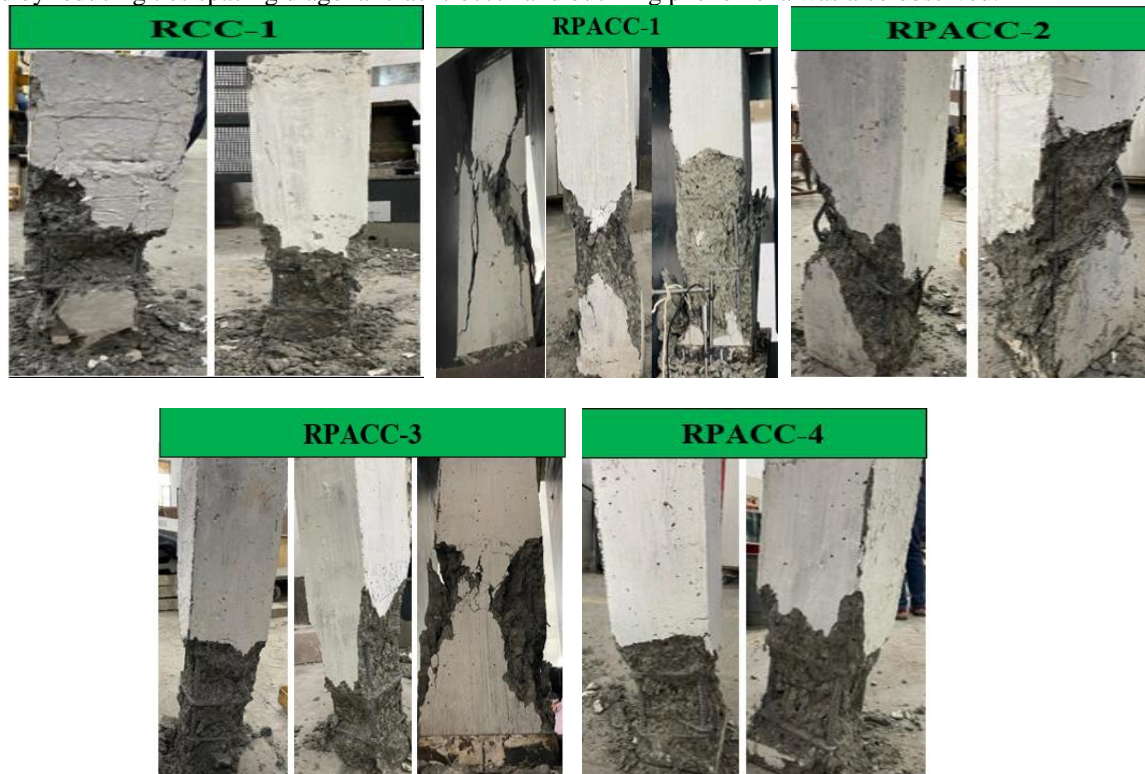
Fig -6: Failure pattern of all column specimen
